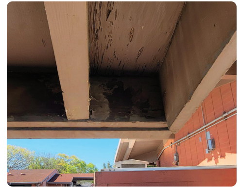
Deteriorating roof at Burchfield Primary School
